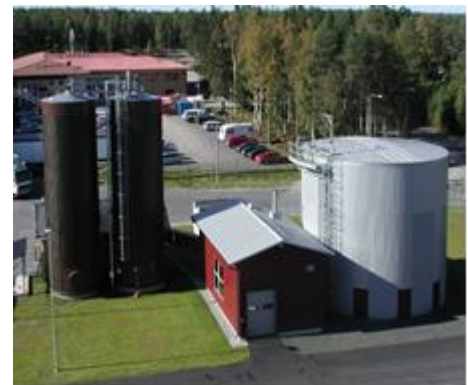
The biological wastewater treatment plant at Norrmejerier in Sweden
