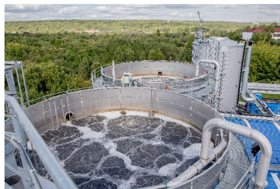
Image: Wastewater treatment at a dairy involves managing many different tasks.
