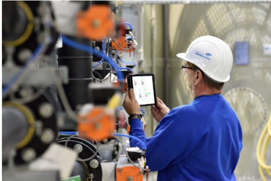
Picture: EnviroChemie's specialist personnel carry out the necessary water technology adjustments during plant management
