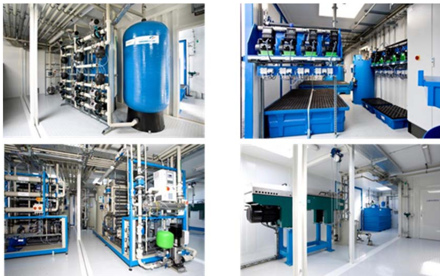
Figure 3. Detail pictures of equipment installed in modules. [Source: EnviroChemie GmbH]
