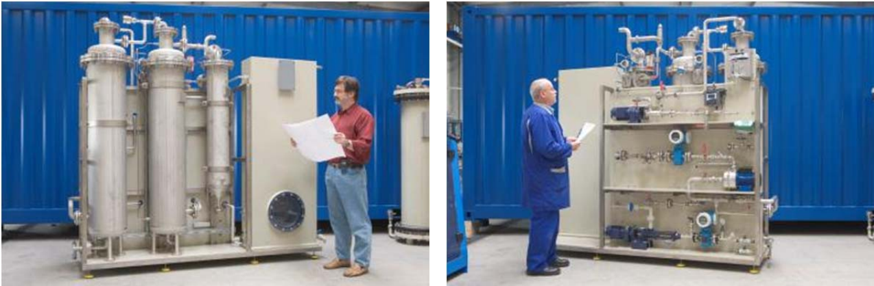
Figure 12. View of the modular ozonation plant during FAT before its installation. [Source: EnviroChemie GmbH]
