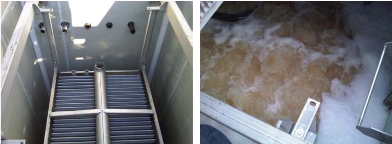
Figure 5. View of ultrafiltration modules (left) and MBR reactor in operation (right). [Source: EnviroChemie GmbH]
