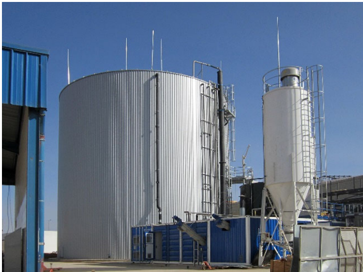
Photo: The sustainable plant solution reduces consumption of resources and operating costs
