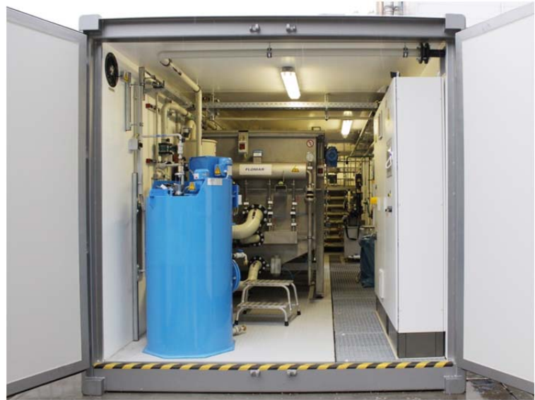
Compact wastewater treatment technology installed in an EnviModul
